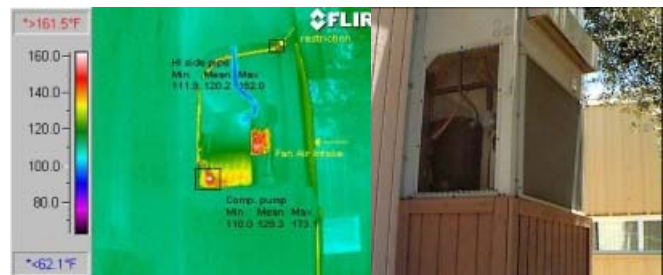
AC unit fault image
