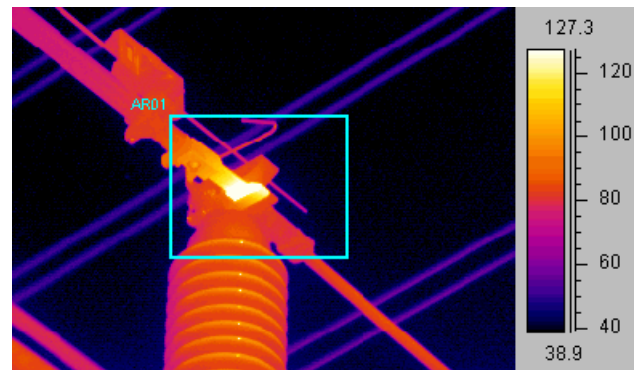
Faulty connection at power station.
